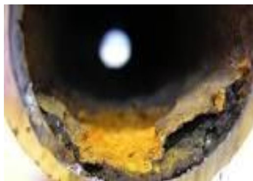
Figure (3): pipeline corroded by H 2 S
